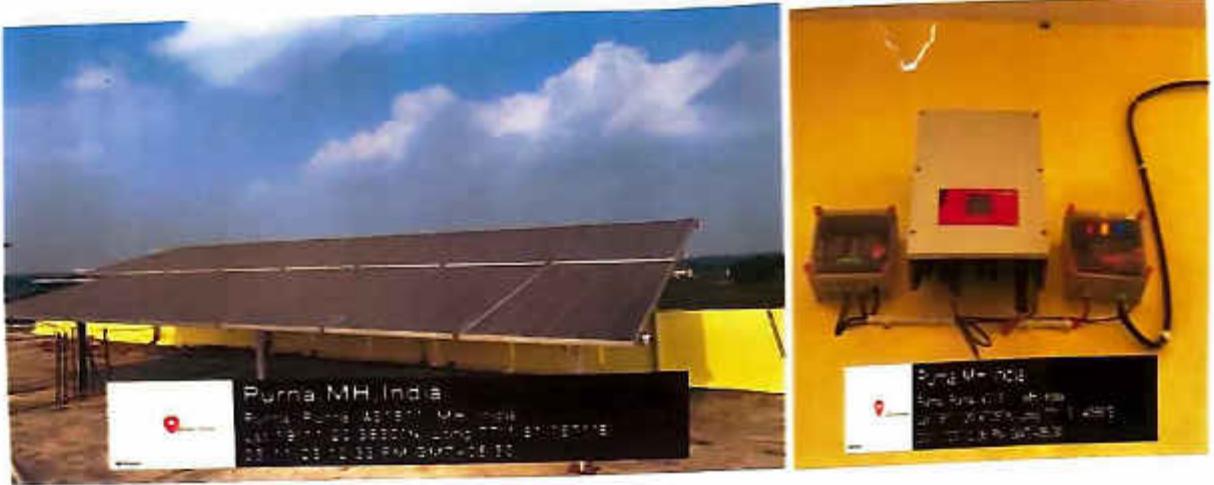
5kw Solar Plant connected to 10 kw inverter
